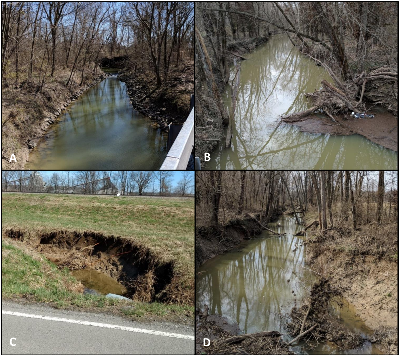
Levels of Eroded Streambanks: A-None or Low (slight); B- Moderate (moderate); C- Severe (high); D- Very Severe (high)
