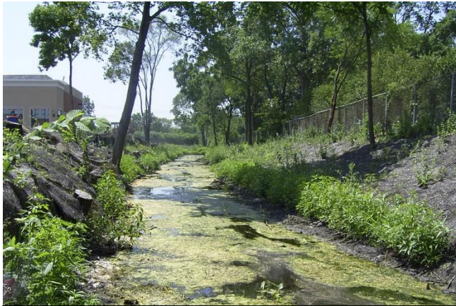
Poor water quality and algal growth along Reach FC10 just west of Route 59
