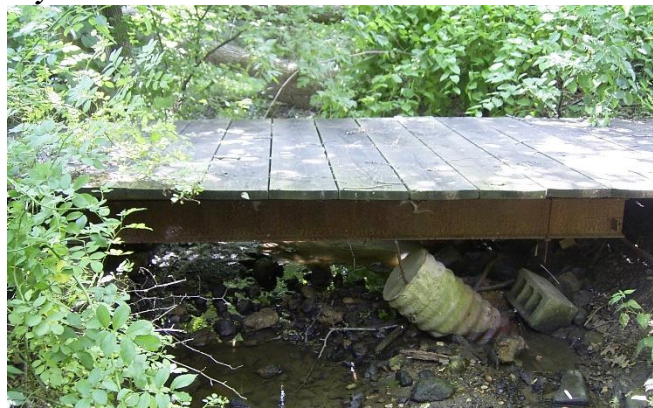
Problematic hydraulic structure (bridge) crossing Reach FC35
