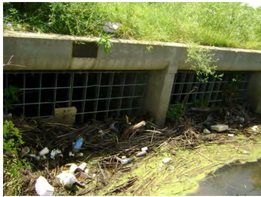
Figure 2-20. Trash and Debris Accumulation and Channel Modification, Frankfort Tributary, Frankfort
