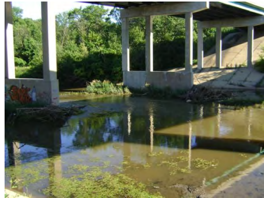
Figure 2-25. Accumulated Sediment and Woody Debris, Hickory Creek at I-80
