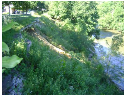
Figure 2-23. Streambank Erosion, Hickory Creek at Hillcrest Road
