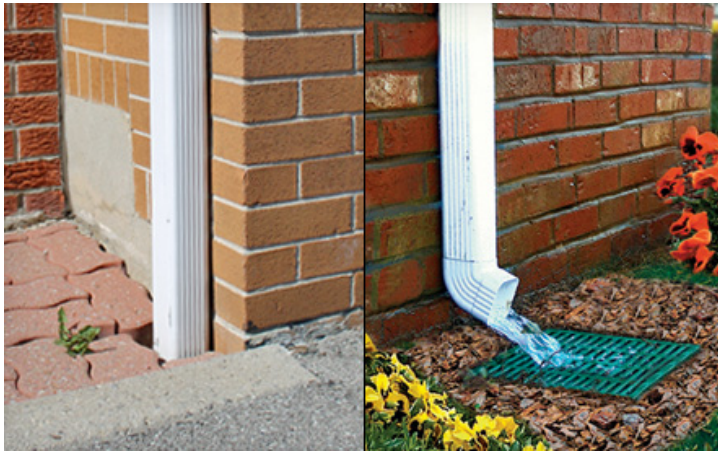
Downspout disconnection, a single property flood reduction strategy. Photo: National Downspout Services.
