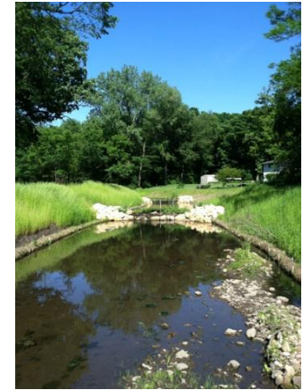
Coir fiber logs with vegetative slopes stabilize streambanks and shorelines in areas with low flow and no wave action (right).
