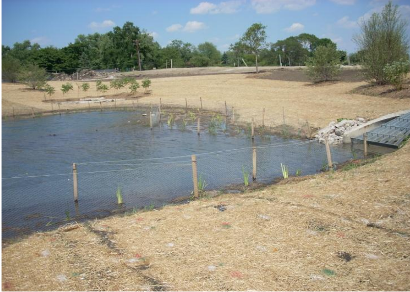
Figure 22: Erosion control blanket used after seeding a newly constructed stormwater detention basin.
