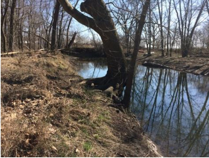
Streambank erosion along south side of bank
