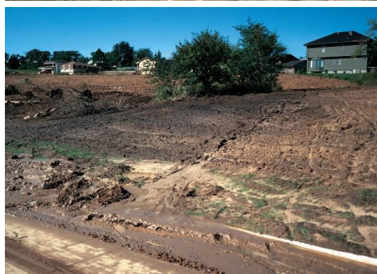
Figure 11. Examples of erosion: Top picture is bank/channel erosion; Bottom picture is sheet and rill erosion.
