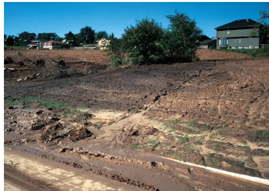
Figure 11. Examples of erosion: Top picture is bank/channel erosion; Bottom picture is sheet and rill erosion.
