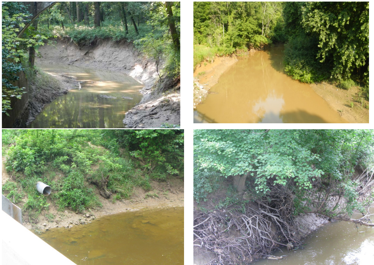
Figure 3-2. Examples of streambank erosion in the Bonpas Creek watershed
