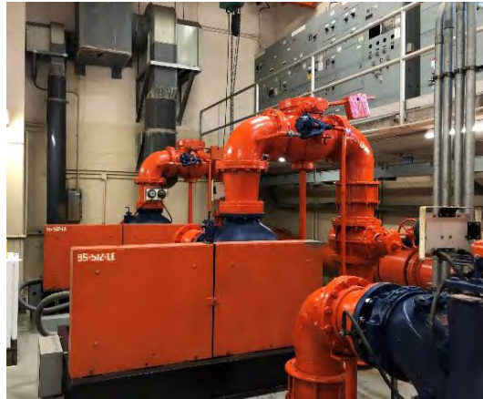
Figure 5-4 Pump Room holding Raw Sewage Pumps
