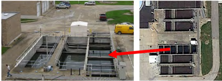
Figure 5-12 Chlorine Contact Tank
