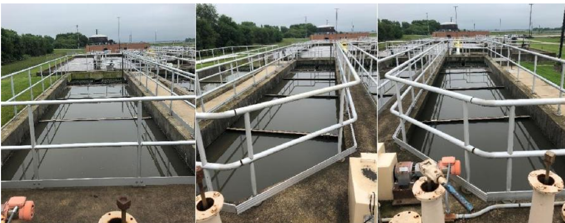
Figure 3-4: East (shown left), Middle (center), and West (right) Primary Clarifiers
