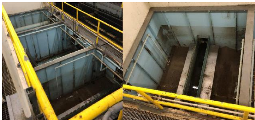
Figure 3-9: Gravity Sand Filters
