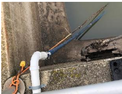
Figure 3-12: PVC pipe used to pump storm water out of the old concentrator infrastructure
