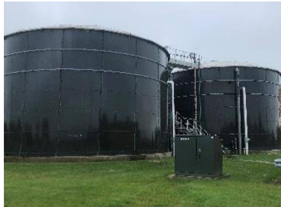
Figure 3-15: Sludge Storage Tanks
