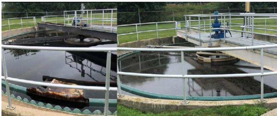
Figure 3-8: Larger Final Clarifier (left) and Smaller Final Clarifier (right)
