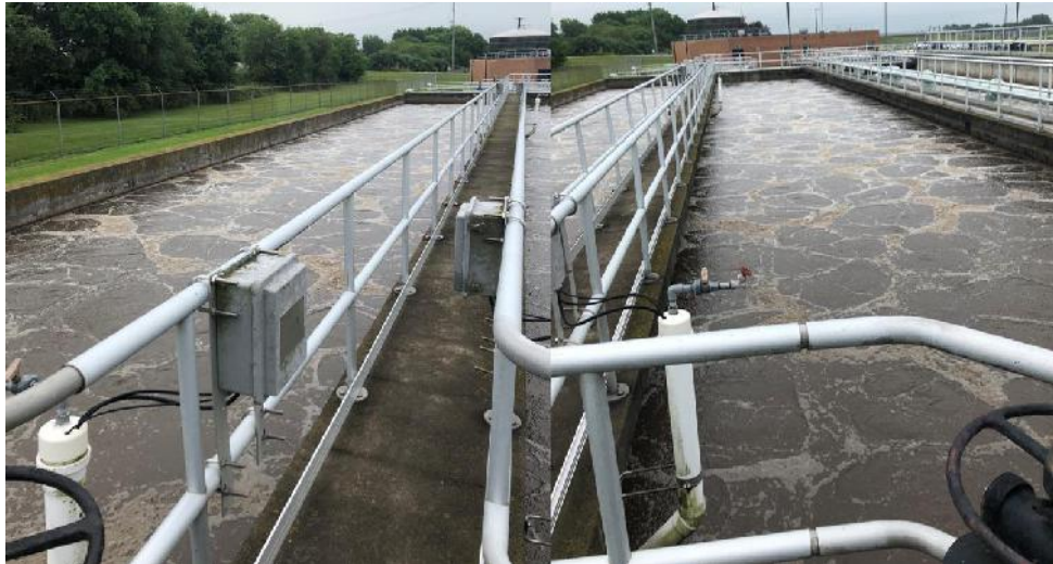
Figure 3-5: East (shown left) and Middle (right) Aeration Basins
