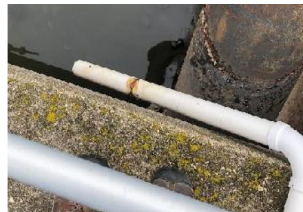
Figure 3-13: PVC Pipe used to discharge the pumped stormwater from the old concentrator to the larger portion of the tank
