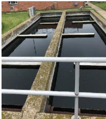
Figure 3-10: Chlorine Contact Tanks
