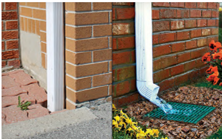
Downspout disconnection, a single property flood reduction strategy. Photo: National Downspout Services.
