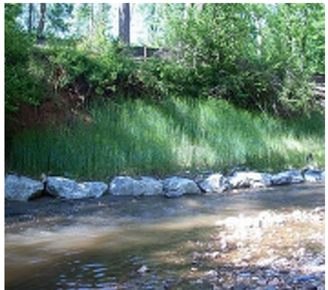
Stone toe protection, which prevents streambank erosion and shoreline erosion. Photo: Montgomery County, Maryland.
