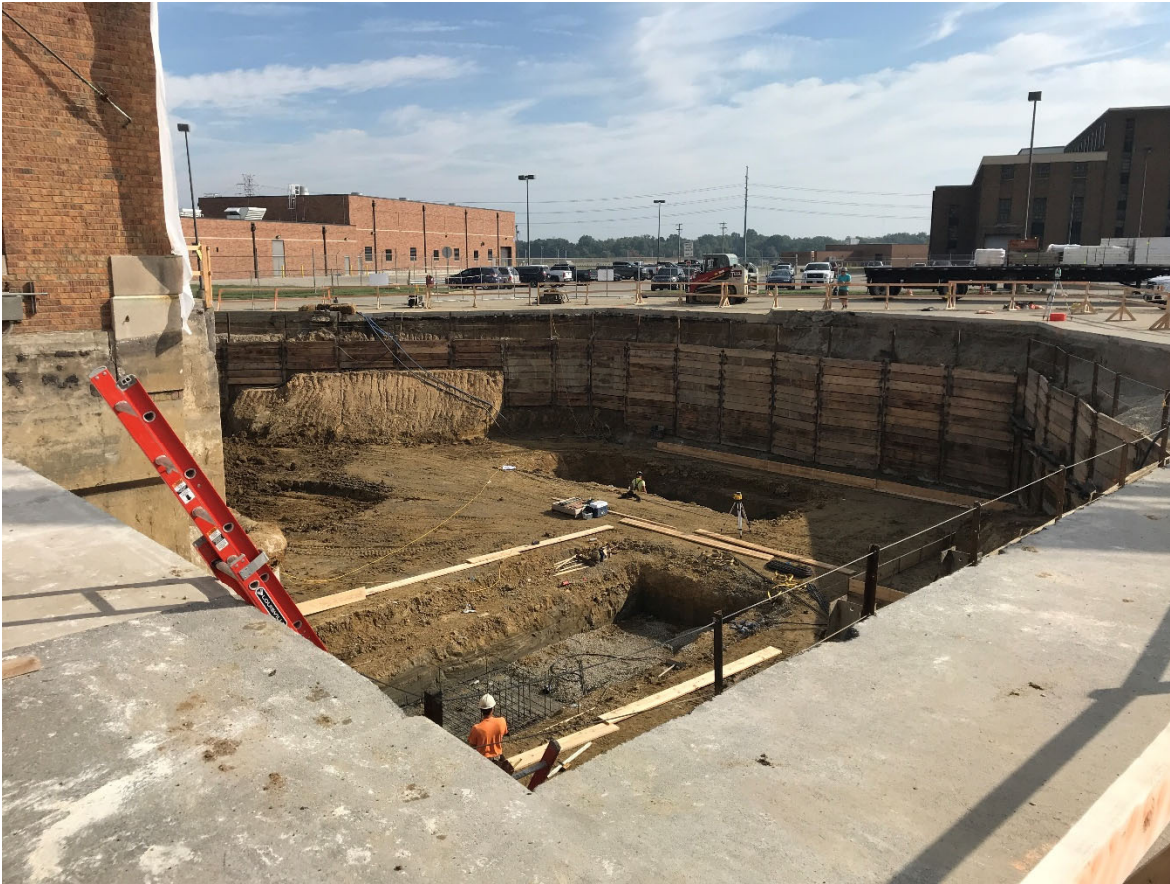
Water Plant Springfield, Illinois
