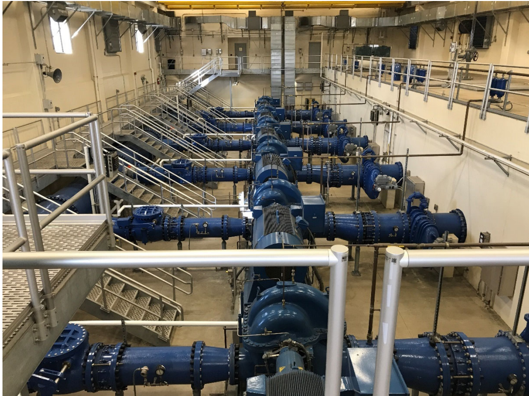
Water Plant Springfield, Illinois
