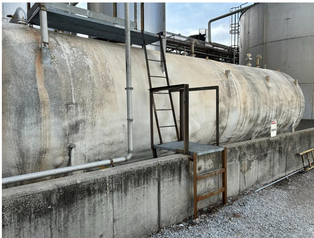
Photo 7 Caustic tank C3
