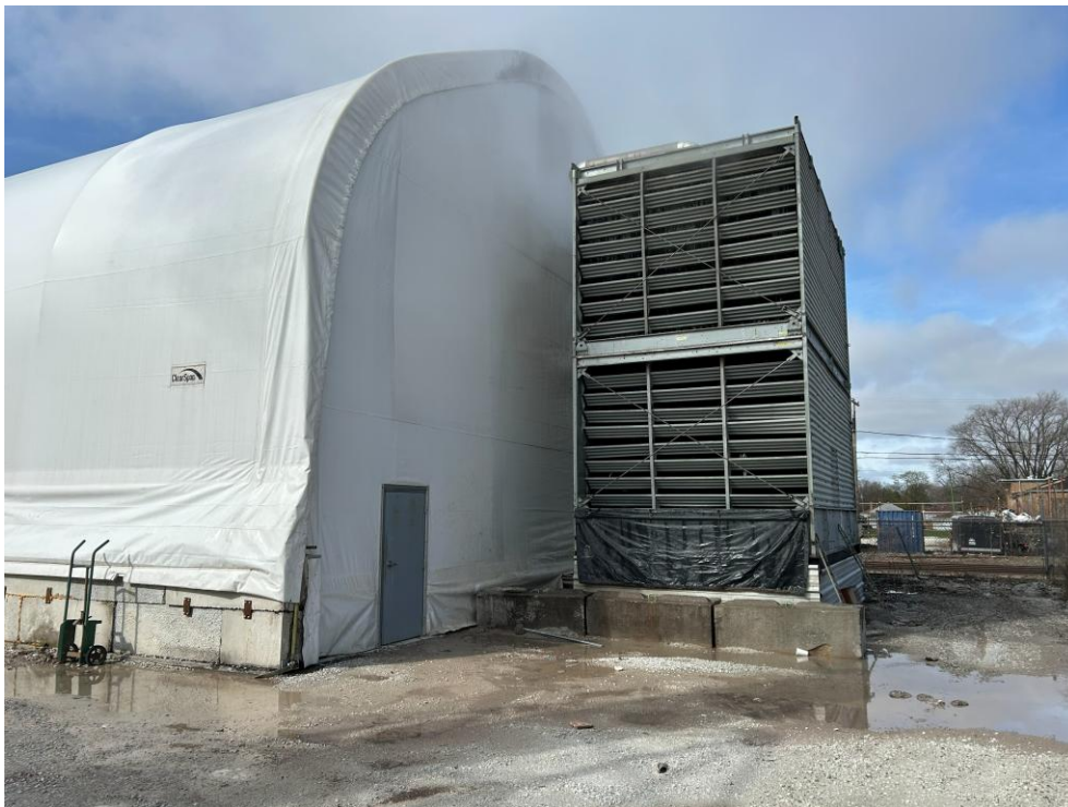
Photo 2: Cooling tower and framed building containing evaporator system
