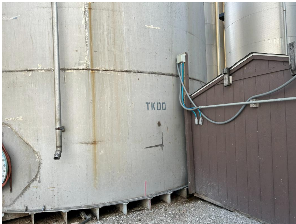
Photo 8 Tank TK00 blended tank wastewater pre and post acidulation
