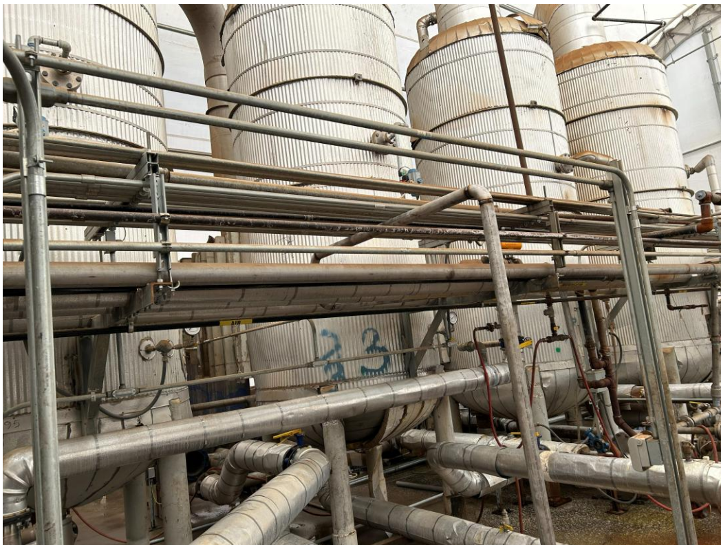
Photo 16: Four Evaporator system units, inside concrete dome building
