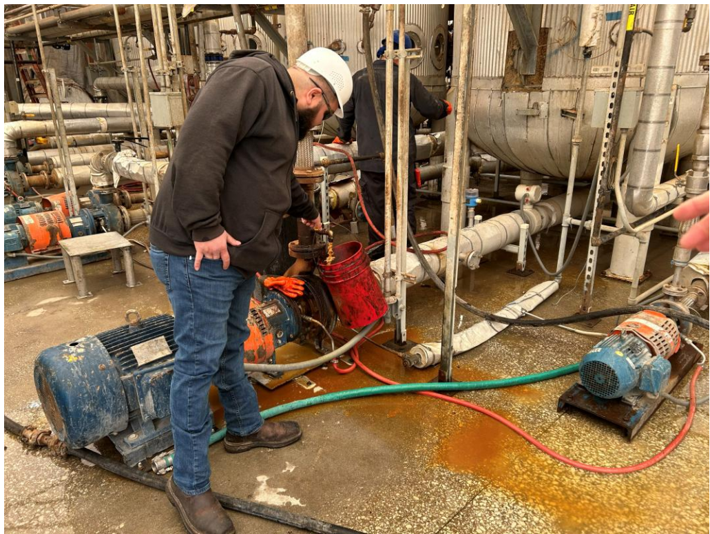
Photo 18 Sample port bucket, pumps, evaporator system
