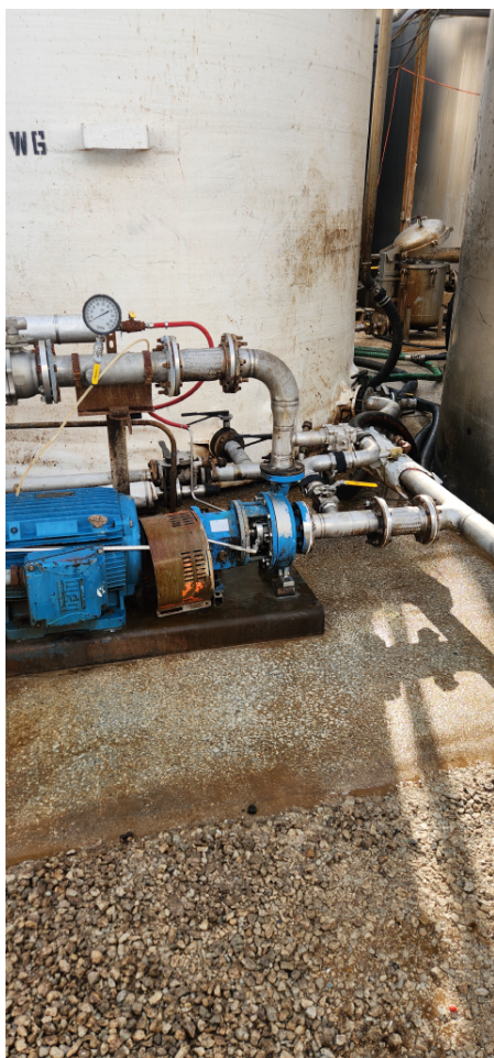
Photo 24 provided from Pullman Innovation 4/8/2026 repaired leak
