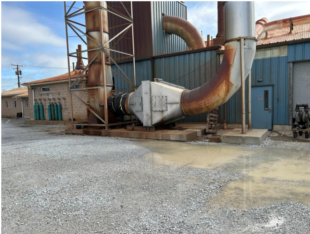
Photo 1: Air control unit, this was where the DAF unit was in the past
