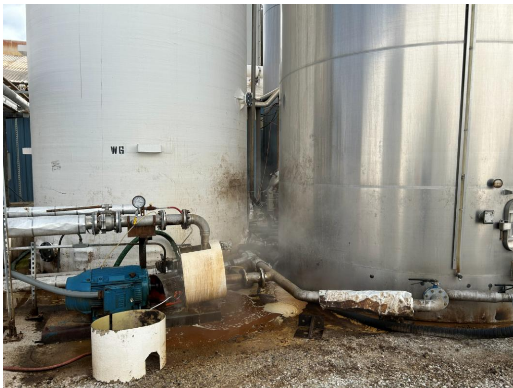
Photo 5: At the time of inspection there was a seal leaking at the flanged connection, this was occurring in front of tank W6. The facility is under combined sewer area
