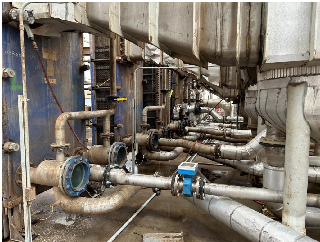
Photo 17: Four Evaporator system units, heat exchangers, inside concrete dome building
