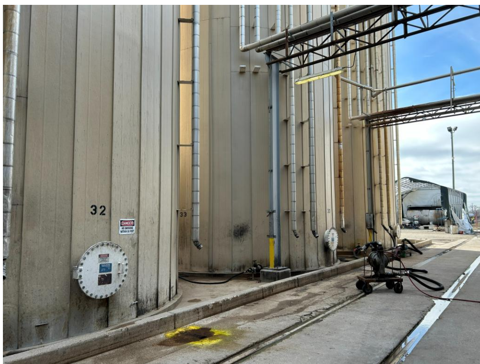
Photo 12 tank area T31 to T34 Advance Acidulation, quick connect hoses with portable pumps
