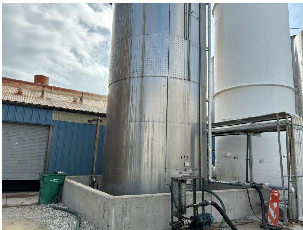
Photo 3: Sludge tank T147
