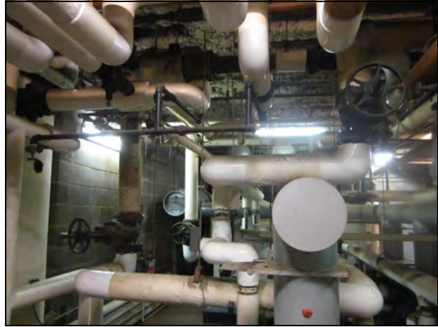
8. View of the piping in the boiler room. All of the TSI appears to be fiberglass and in good condition.
