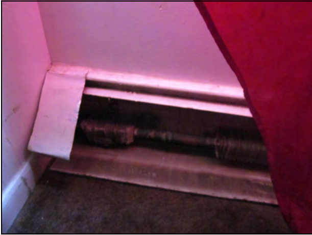
37. View of a typical unit baseboard heater. No insulation was observed.
