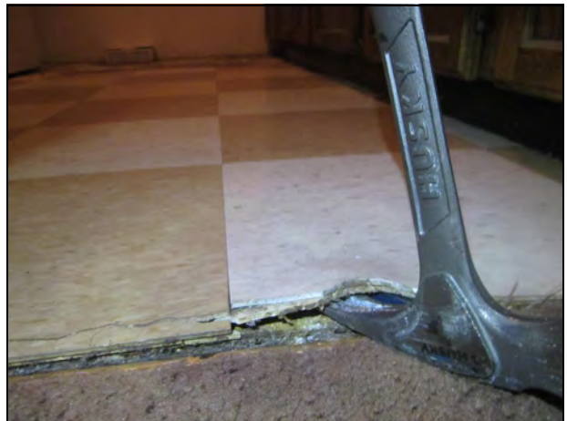
28. View of a typical kitchen floor system. Two layers of tile over plywood, on top of concrete.
