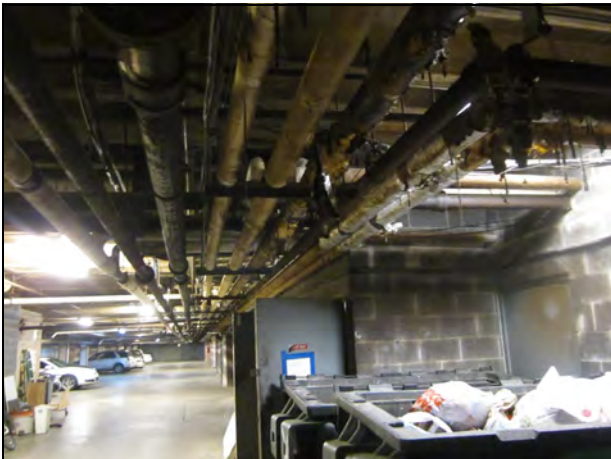
11. View of the pipes in the garage running along the ceiling.
