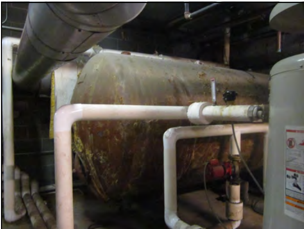
5. View of the hot water holding tank. Bits of fiberglass insulation are stuck to the tank.
