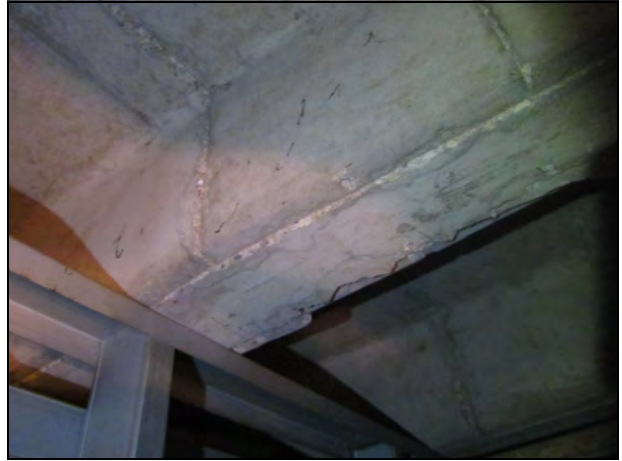
32. View inside the hatch showing concrete without spray-on fireproofing.
