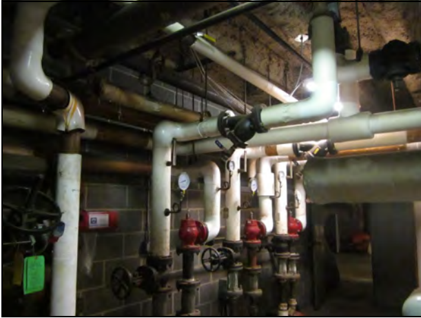
7. View of the piping in the boiler room. All of the TSI appears to be fiberglass and in good condition.
