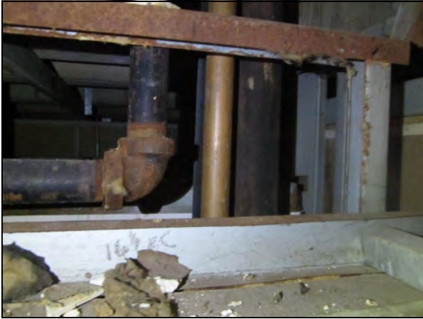
31. View inside the hatch revealing non-insulated pipes.
