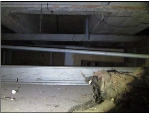
33. View inside the hatch of an insulated duct (could not be sampled) probably for bathroom/kitchen exhaust.
