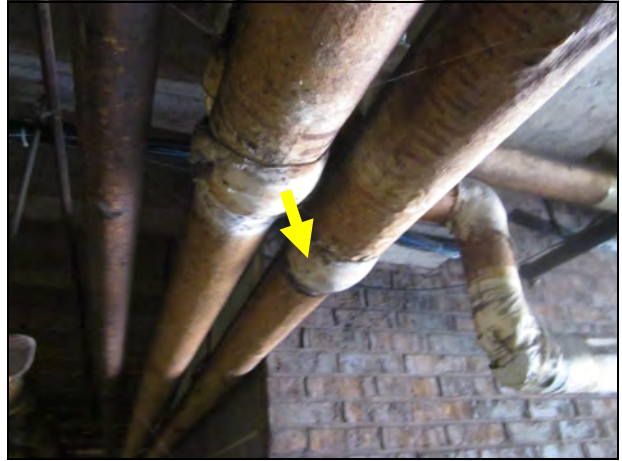
14. View of TSI joint Sample #6, near the elevator equipment room. The pipe run TSI is fiberglass.
