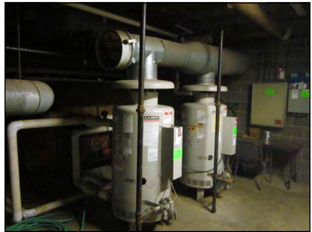
4. View of boiler room equipment. The TSI all appears to be fiberglass and in good condition.
