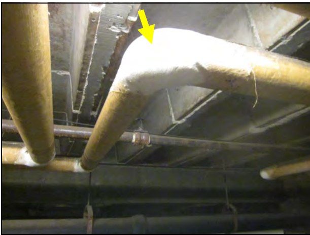
15. View of TSI joint Sample #7, near parking spot #10. The pipe run TSI is fiberglass.
