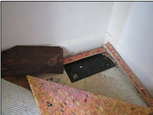
23. Close-up of the previous photo. The red tile is on the left, the black mastic is on the right. The white is either paint or leveling compound.
