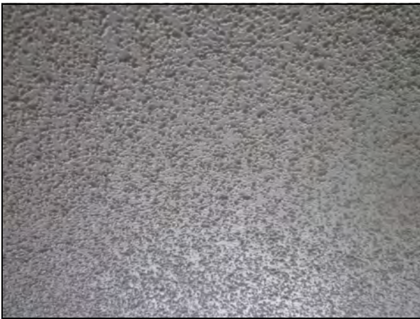
21. Close-up of the texture surfacing material present on the ceilings. The material is applied to gypsum board.
