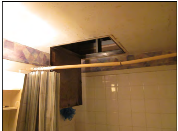
30. View of a ceiling hatch in the bathroom of a unit.
