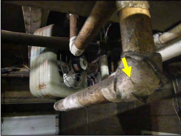
13. View of TSI joint sample #5, near the roll-up garage door. The pipe run TSI is fiberglass.
