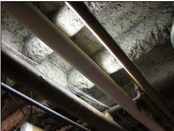
9. View of the spray-on fireproofing on the concrete ceiling of the boiler room.
