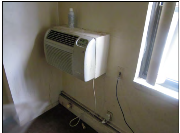
36. View of a typical through-wall A/C unit.
