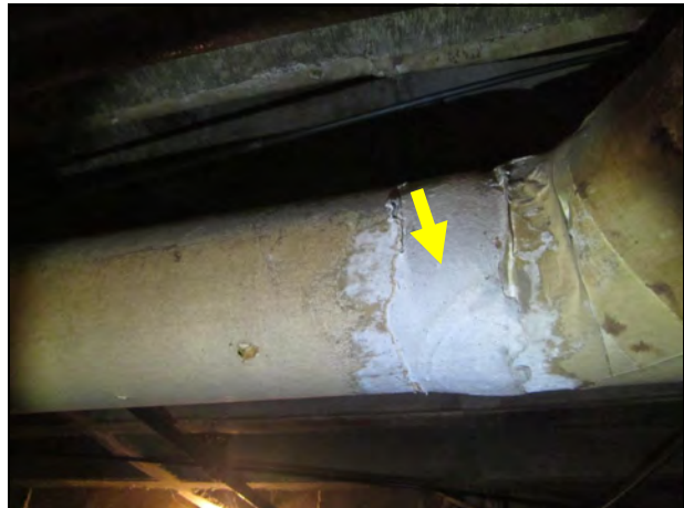
12. View of the TSI joint: Sample #4, near parking spot #34. The TSI on the pipe run is fiberglass.
