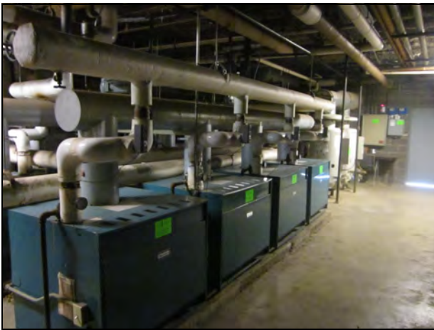
3. View of the boiler room. The TSI all appears to be fiberglass and in good condition.
