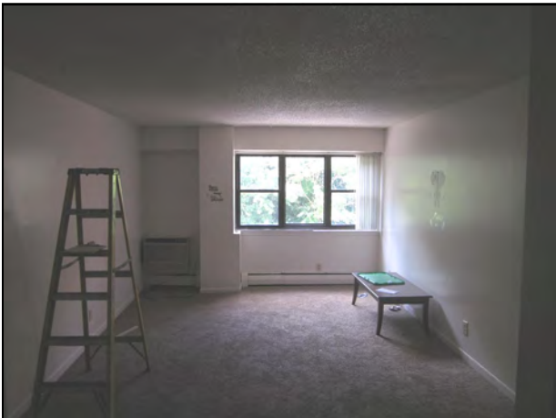
17. View of a typical Living Room; note the textured ceiling, and gypsum board (drywall) throughout.
