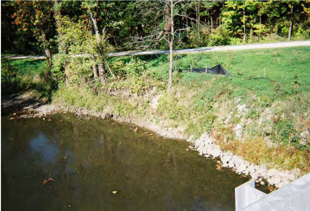
Photograph No. 7 Orientation: Northeast Description: Failed silt fencing along east bank of Salt Fork Creek (Field book photo # 7)
