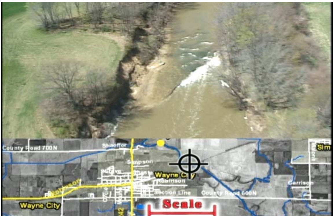
Fig. 24 Exposed bedrock in Skillet Fork is a geologic control preventing headcut from advancing upstream.
