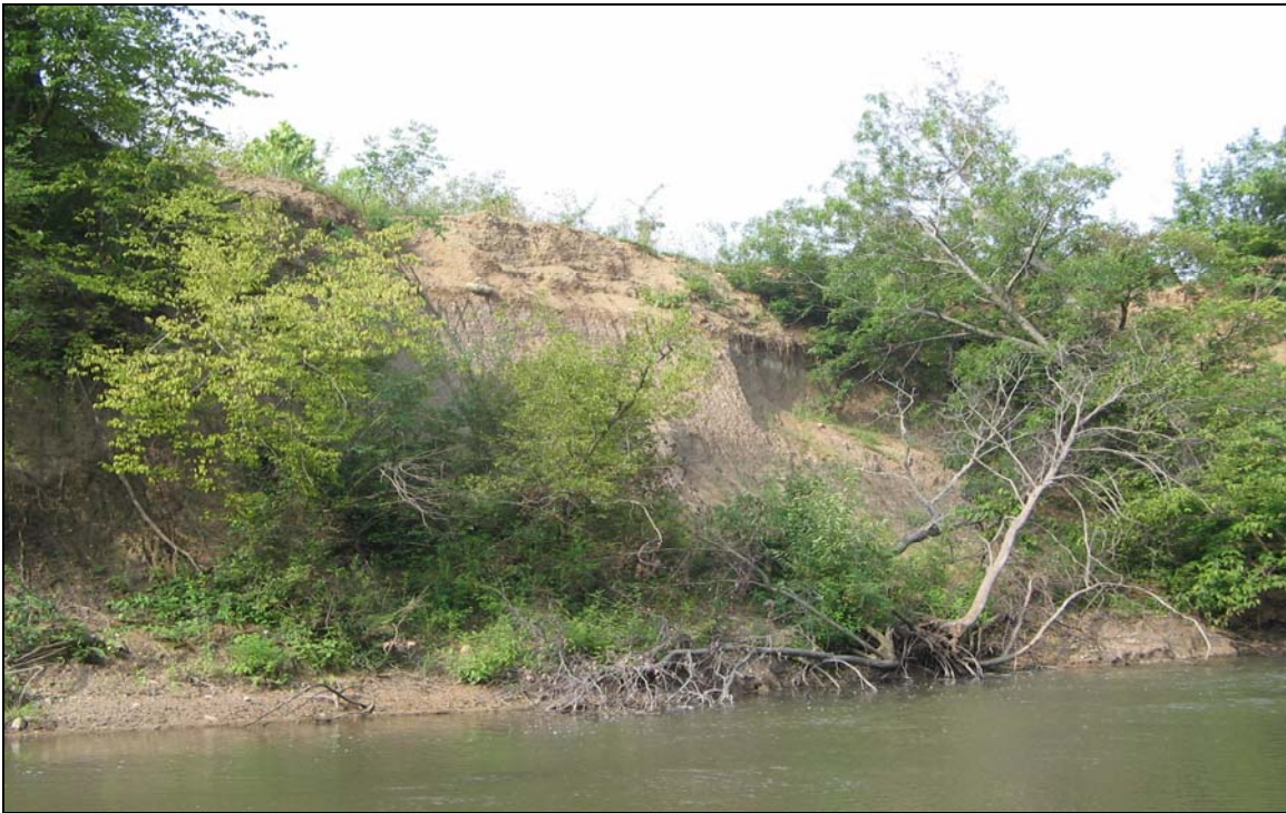
Fig. 6 Eroding escarpment near Cross Section 1 resulting from toe scour.
