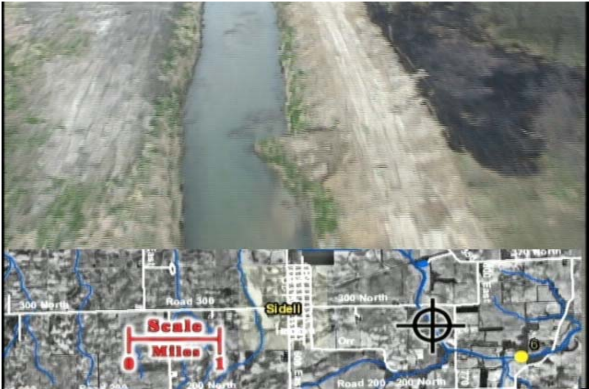
Fig. 13 Slumped bank; geotech failure possible caused by improper bank shaping
