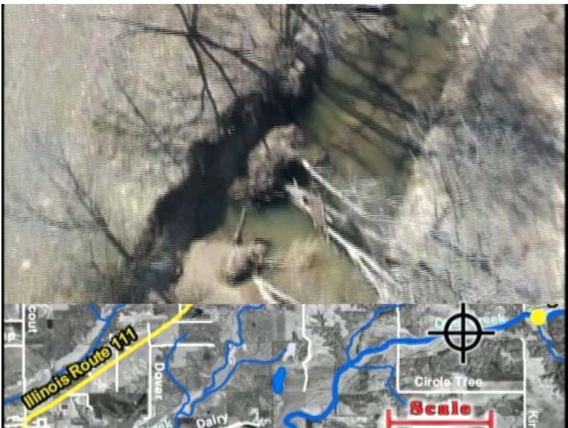
Failing banks in Chapter 3 causing mature trees to collapse into channel
