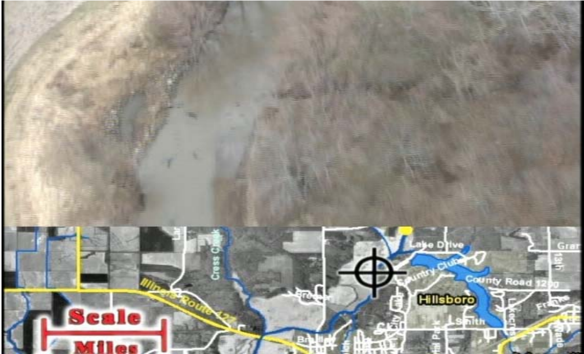
Fig. 8 Stone Toe Protection installed around 1998 for lateral bank treatment. Note the stable banks and ponded water behind the STP in the apex of the bend.
