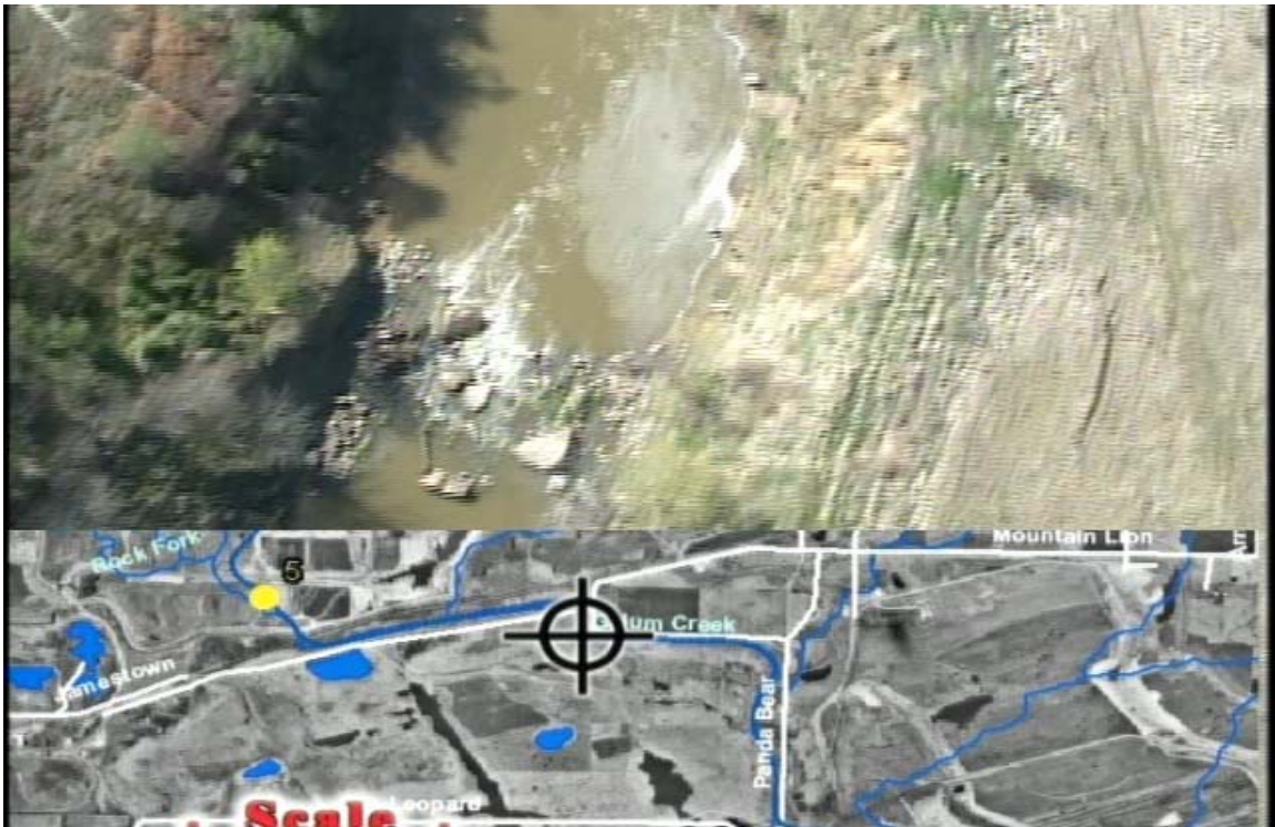
Fig. 17 Grade Control Structure Needing Maintenance at DVD Disc 1 26:30
