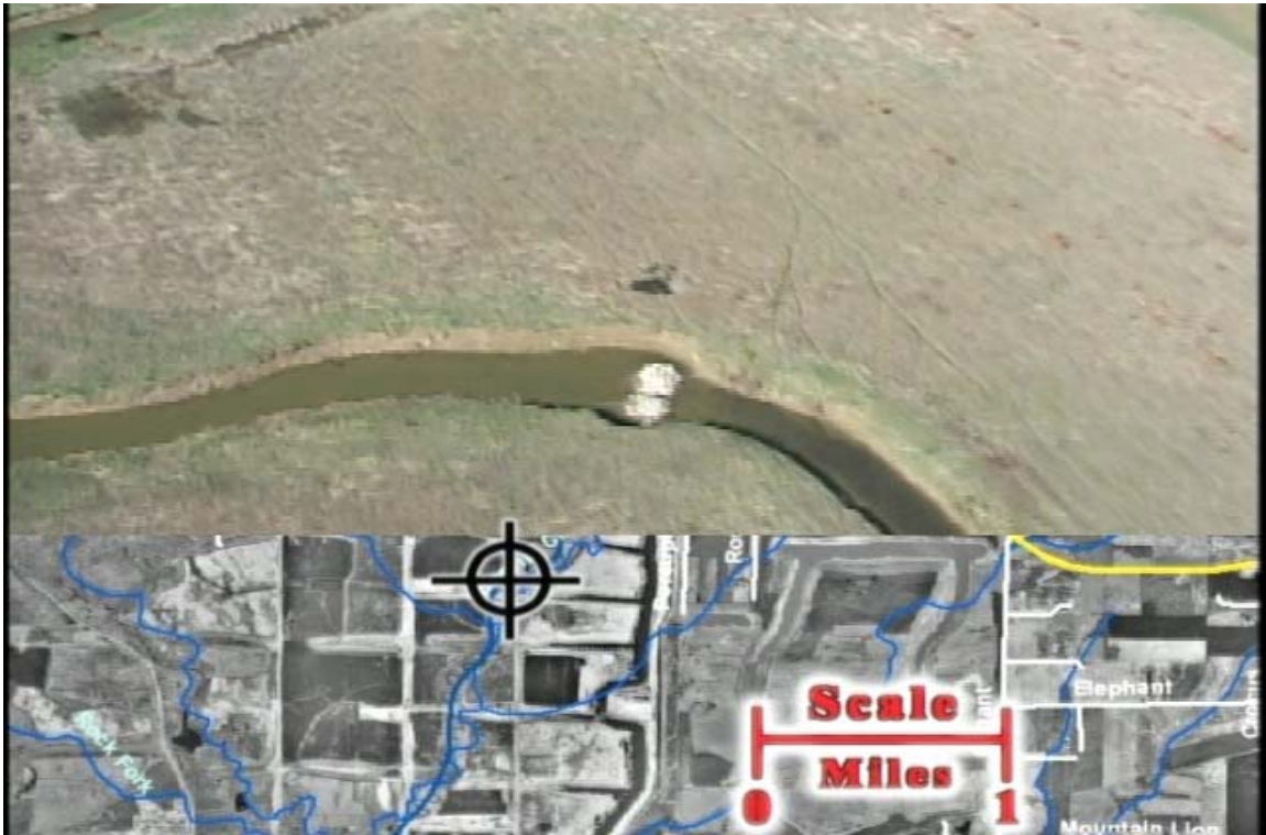
Fig. 14 Failed Grade Control Structure in reclaimed mine land. DVD Disc 1 at 22:37
