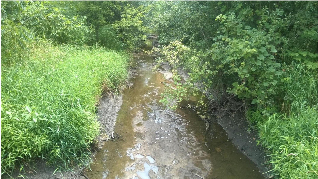
Figure 35 Erosion along Winfield Creek
