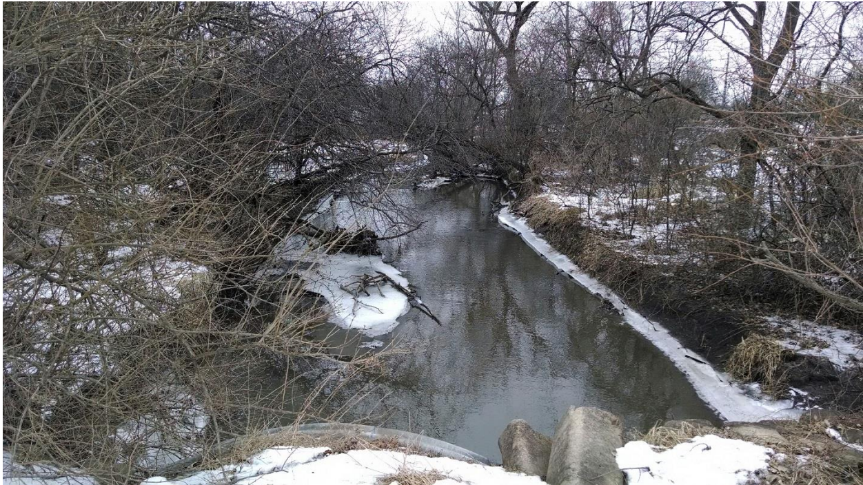
Figure 33 Eroded streambanks along Kress Creek
