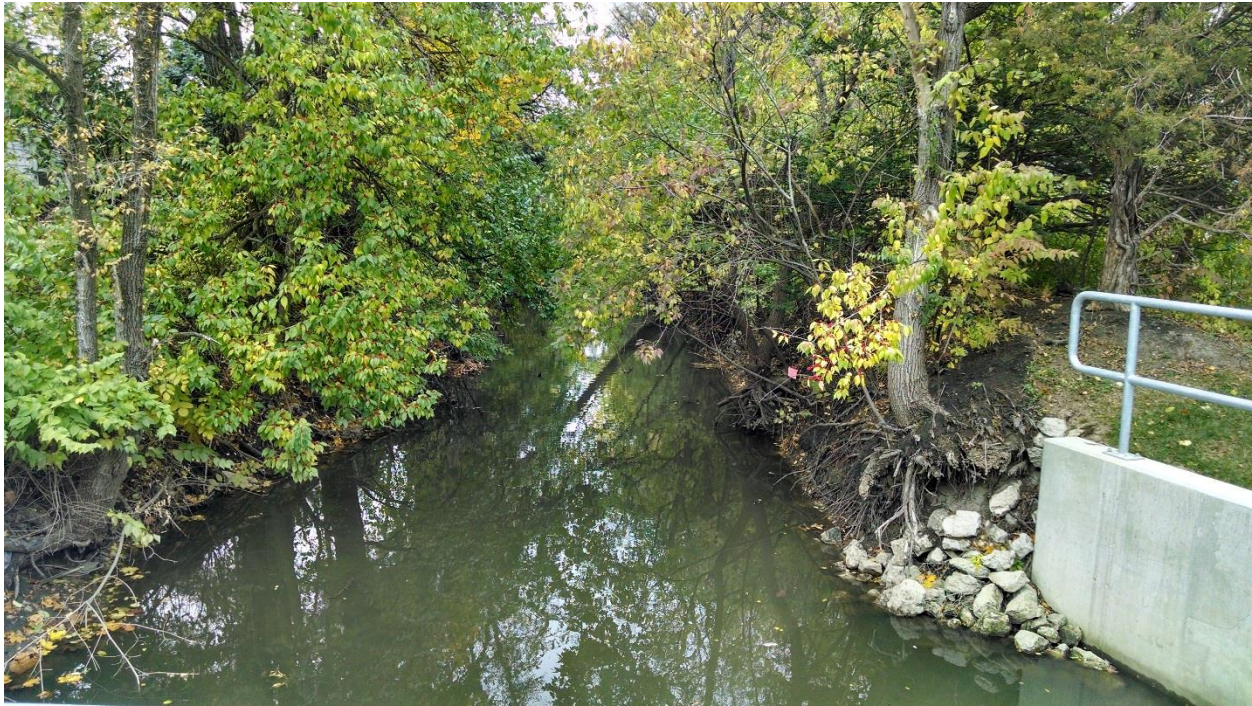
Figure 34 Erosion along Klein Creek near Hiawatha Drive in Carol Stream
