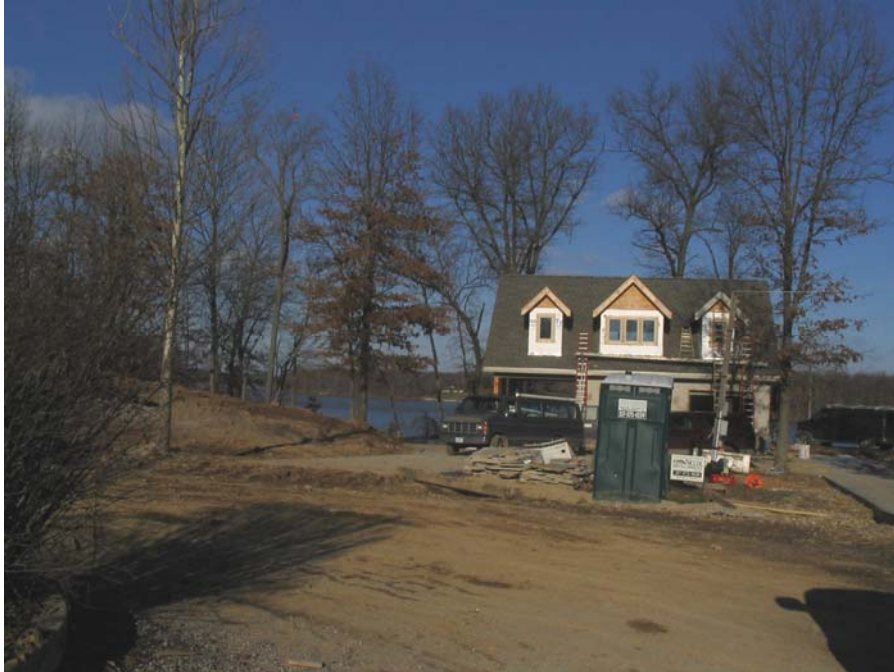
New construction in subdivision (note lack of soil erosion controls)
