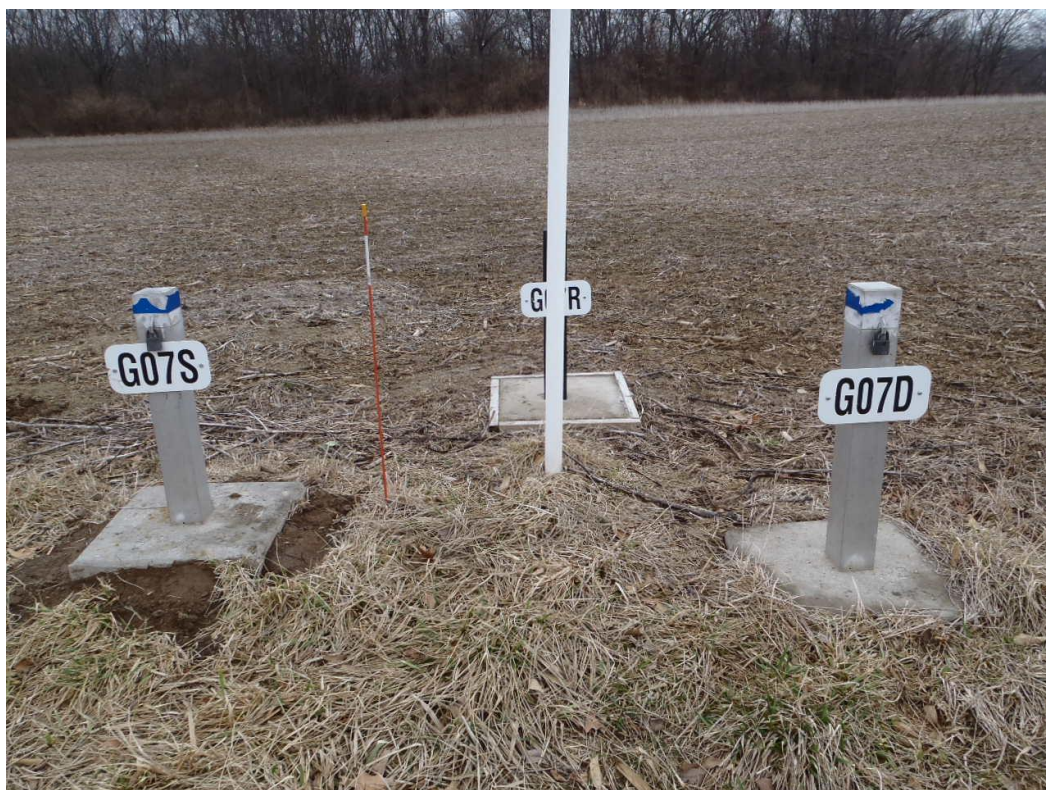
Date: 4/2/2014 Time: 11:23 A.M. Direction: West Photo by: Jeff Turner Exposure #: 046 Comments: G07 cluster; white pipe is visibility marker. Well behind white pipe is G07R.
