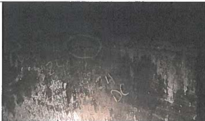
Description: 3 arc gouged areas at tray level 24. Depth as marked
