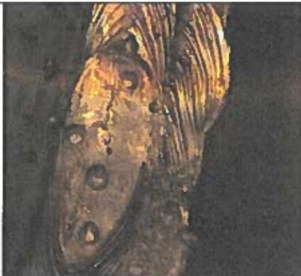
Description: Dehyd Vapor nozzle N4 fillet weld crater crack
