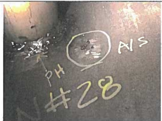
Description: N28 pin hole with crack and arc strike area. .030" depth of arc strikes
