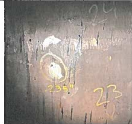
Description: Shell defect areas above tray 23 @ xxx degrees
