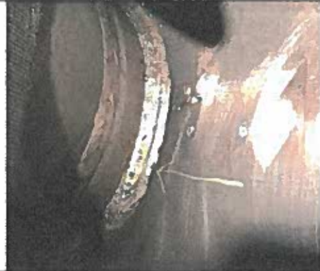
Description: Dehyd Vapor nozzle N 4 fillet weld crater crack, arc strikes
